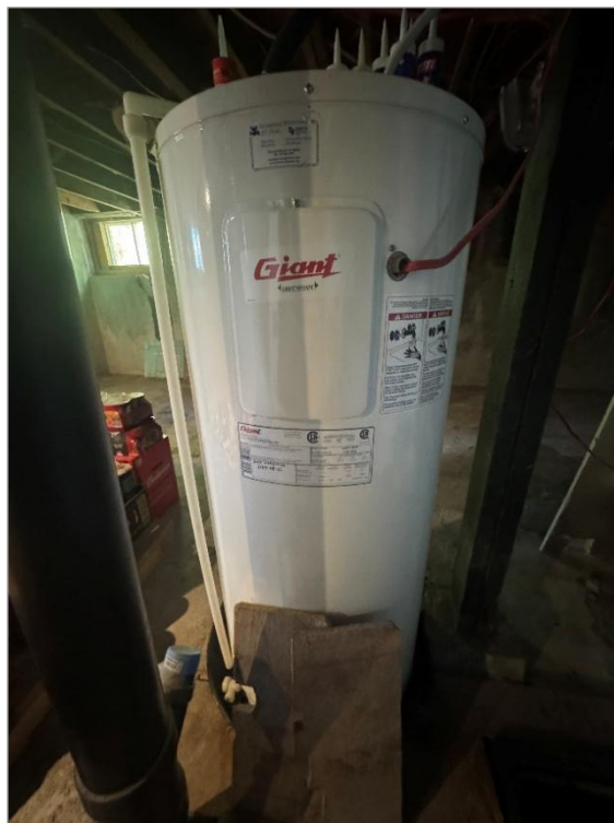
Hot water tank
