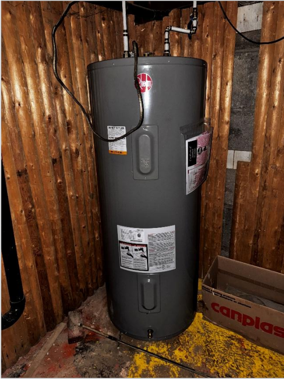
Hot water tank
