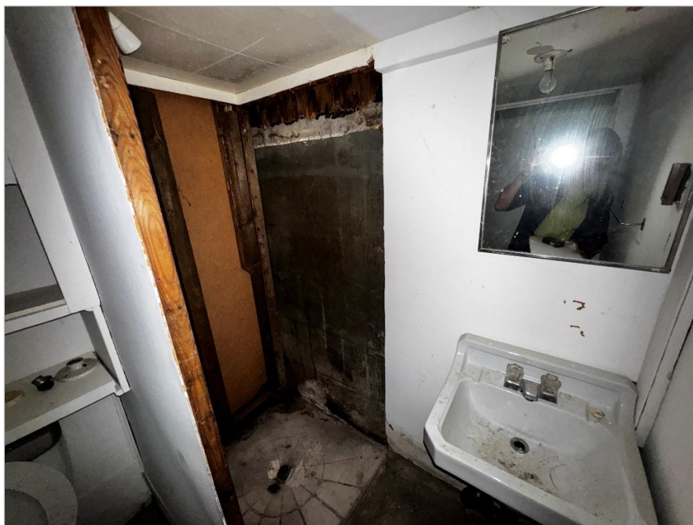
Non-functional basement bathroom
