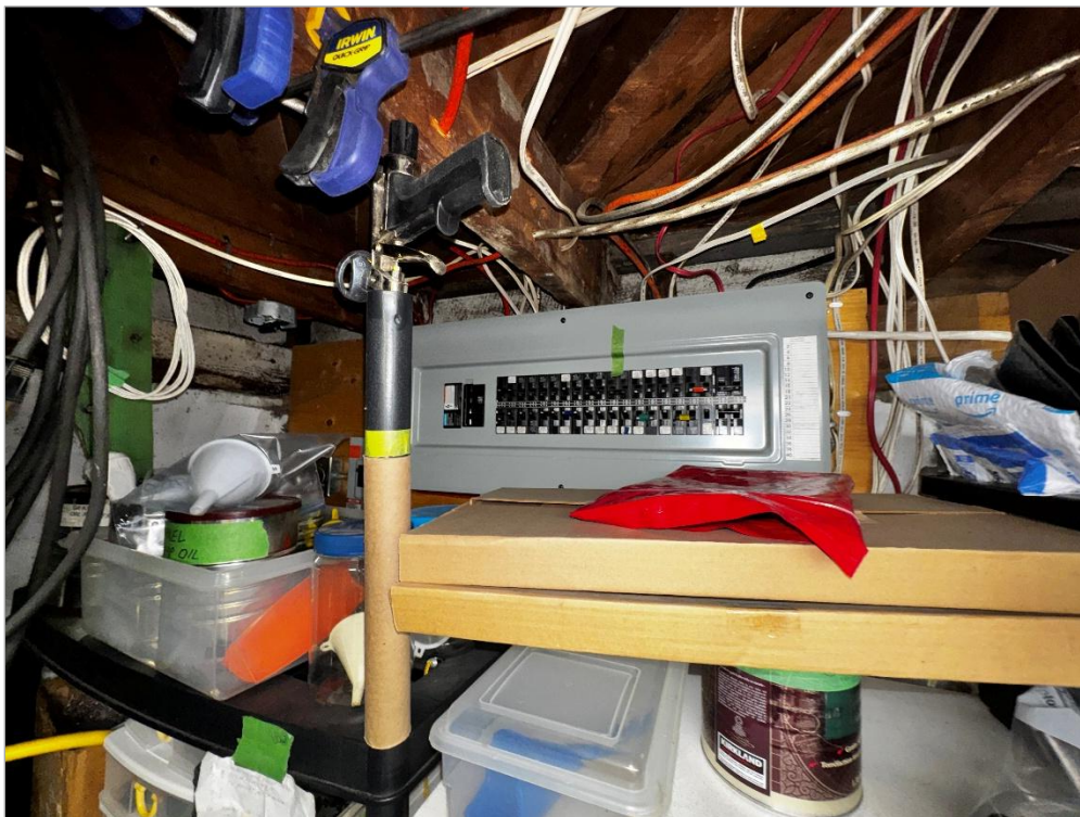
Electrical panel (basement)
