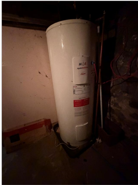
Hot water tank
