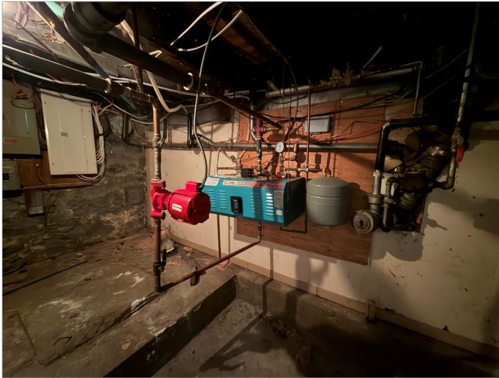
Hot water heating system
