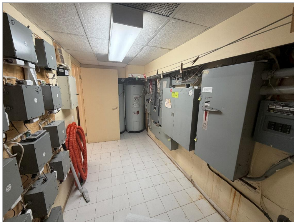
Electrical and mechanical room
